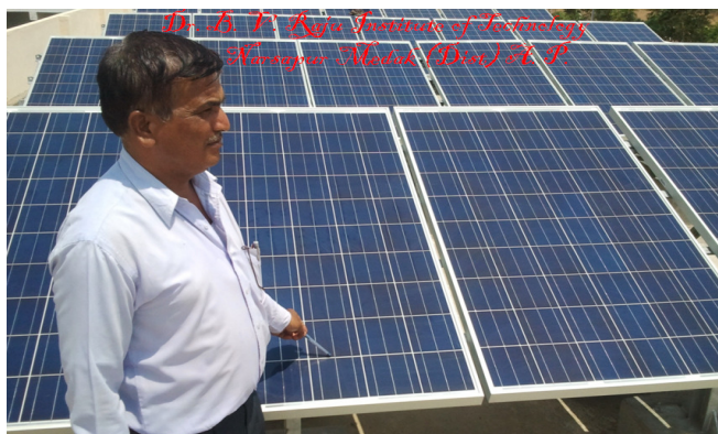
Fig. 1. Solar arrays stationary setup.
